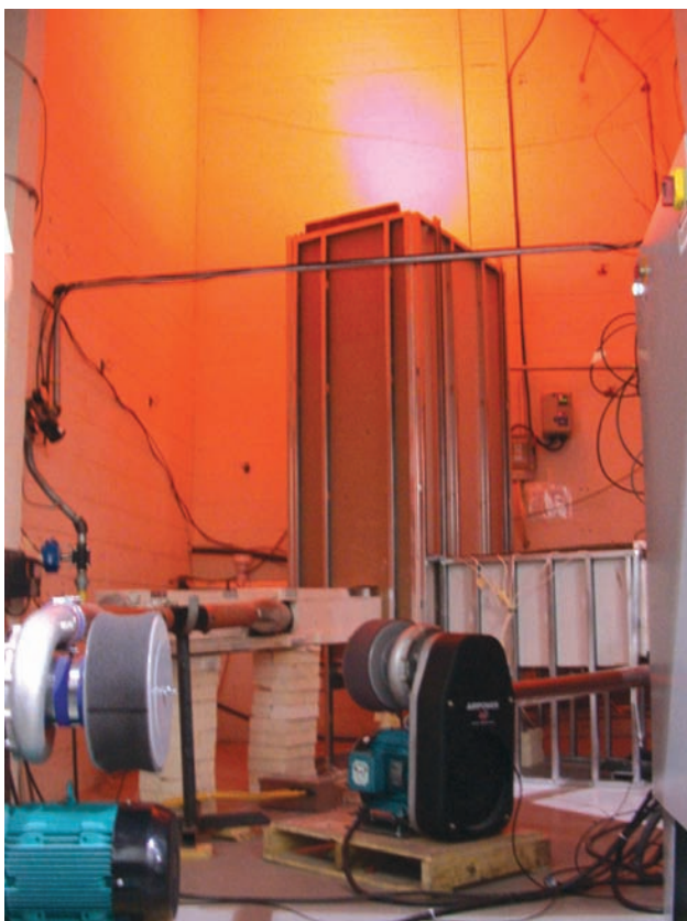
FIGURE 2. HGM-10,000 Burner Test Setup
