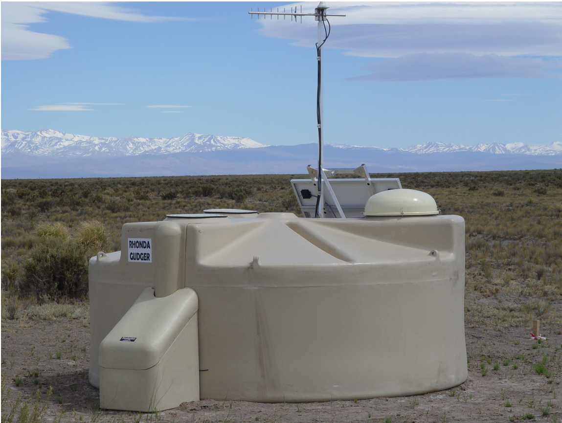
Figure 2.15: Surface detector station for the Engineering Array showing the battery box in place.
