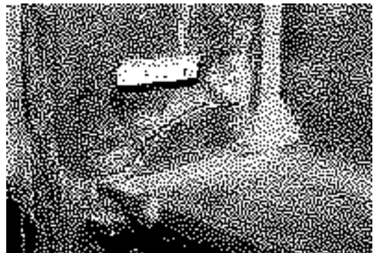
b. Column Flange "Divot" Fracture
