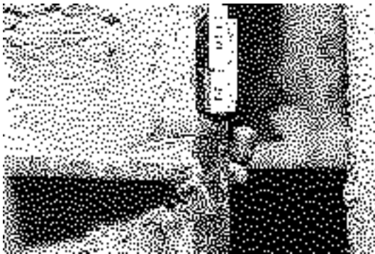
a. Fractures through Column Flange
