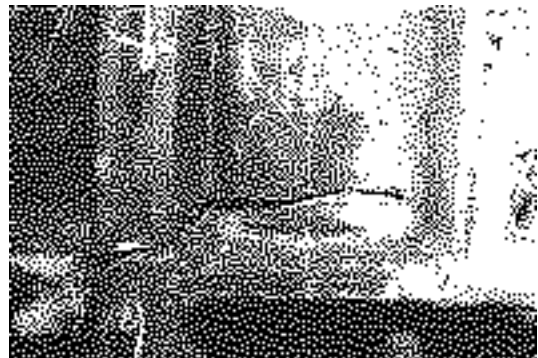
b. Fracture Progresses into Column Web
