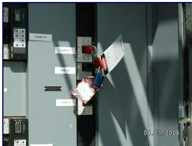
Figure 2.1. 331 Building, CHWP #1 and #2 Breaker, Labels
