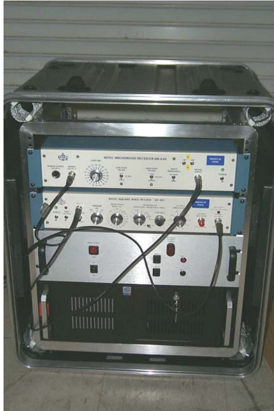
Figure 6.2. SRAIV-SAFT Tank Top Enclosure
