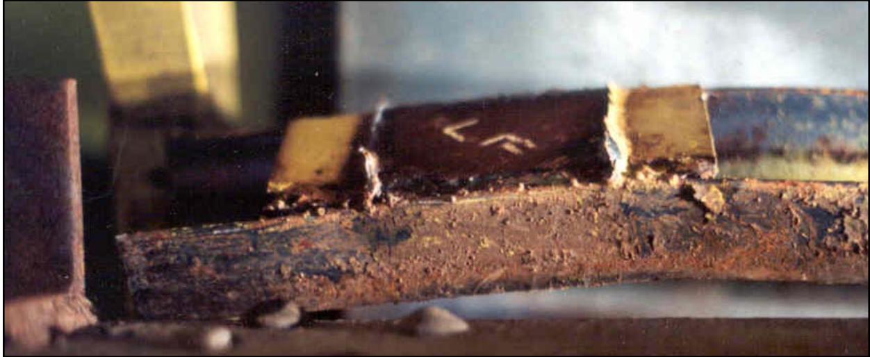
Photo 5. Tank frame at bracket location; weld material remains on tank frame
