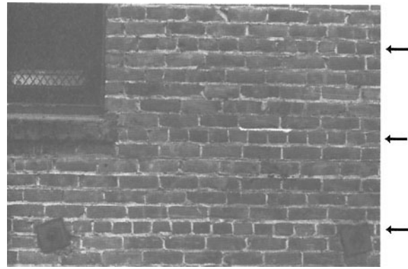
Figure D-10 URM wall showing header courses (identified by arrows) and two washer plates indicating wall anchors.
