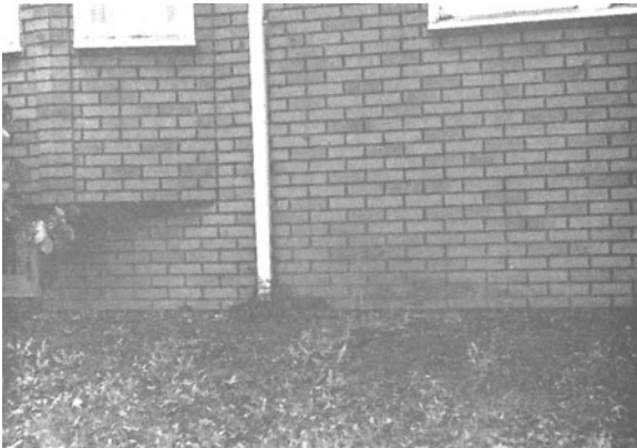
Figure D-16 Asphalt siding with brick pattern.
