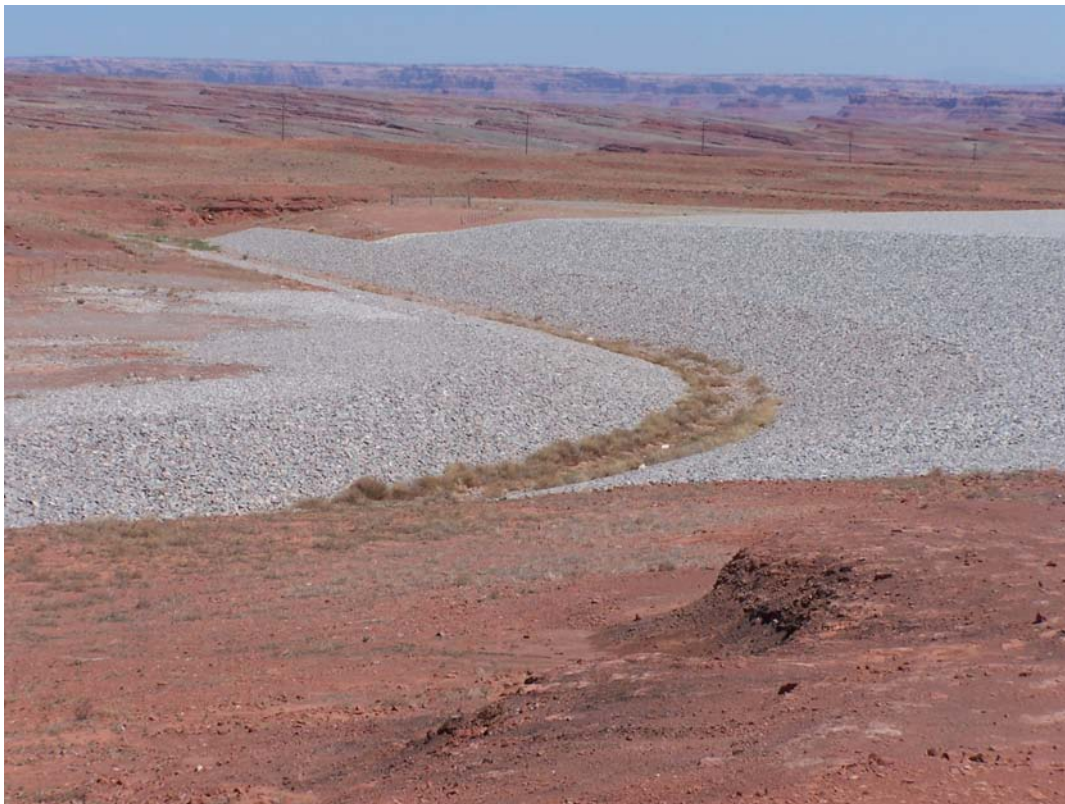
HAT 4/2065. PL-4. Sediment and vegetation in the upper reach of the west diversion channel.
