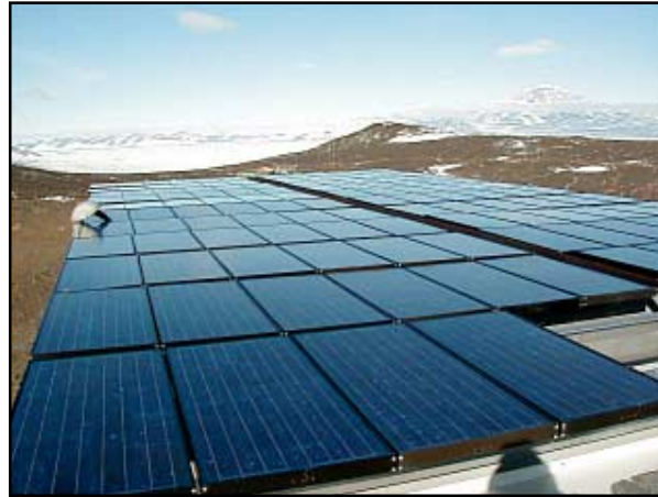
A bank of solar panels soaks up the sun on Black Island. Photo by Frank Howell.
