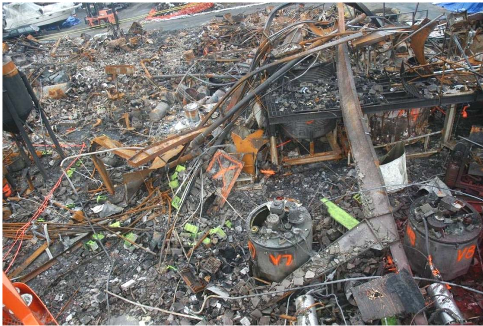
Figure 17. Debris from shattered CMU walls and collapsed roof trusses in area C.
