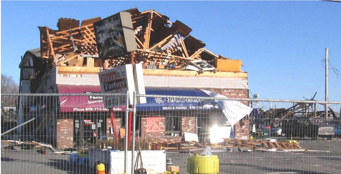
Figure 12. Bakery/pizzeria building destroyed by the explosion (CAI/Arnel building far rear on right).
