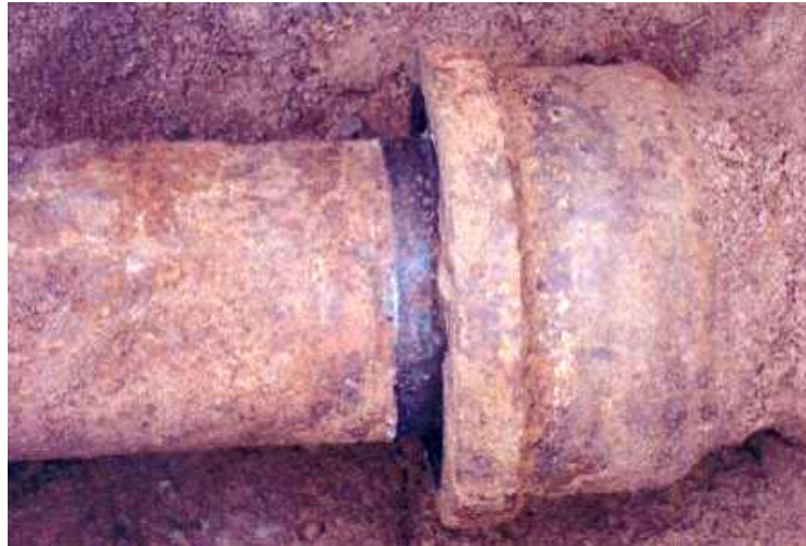
Figure 19. Old 4-inch cast iron buried gas distribution bell and spigot pipe joint partially separated by the explosion (KeySpan photo).
