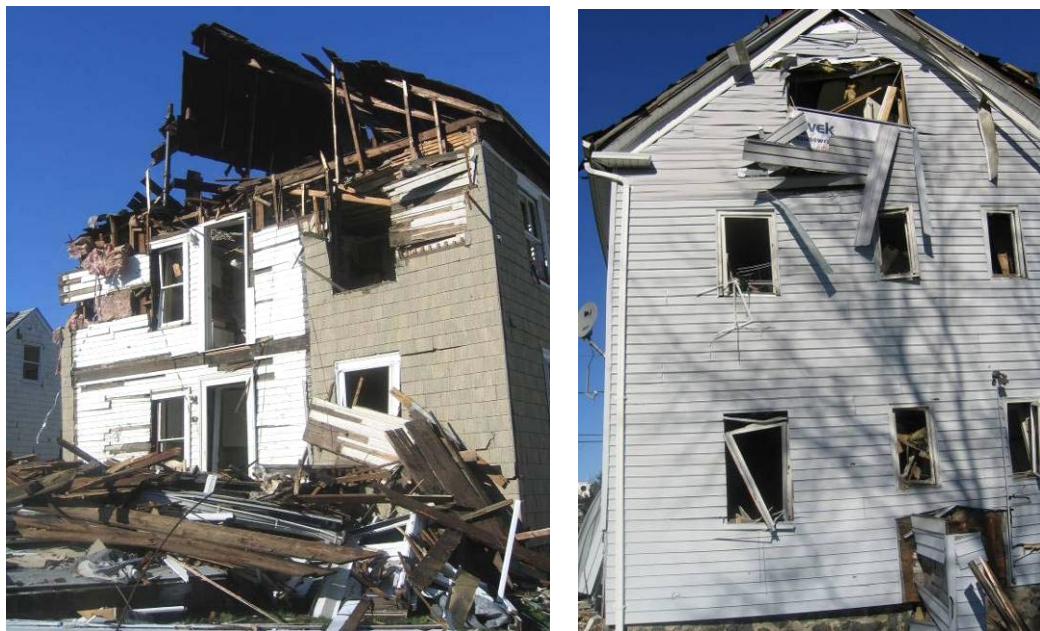
Figure 11. Houses destroyed by the explosion.
