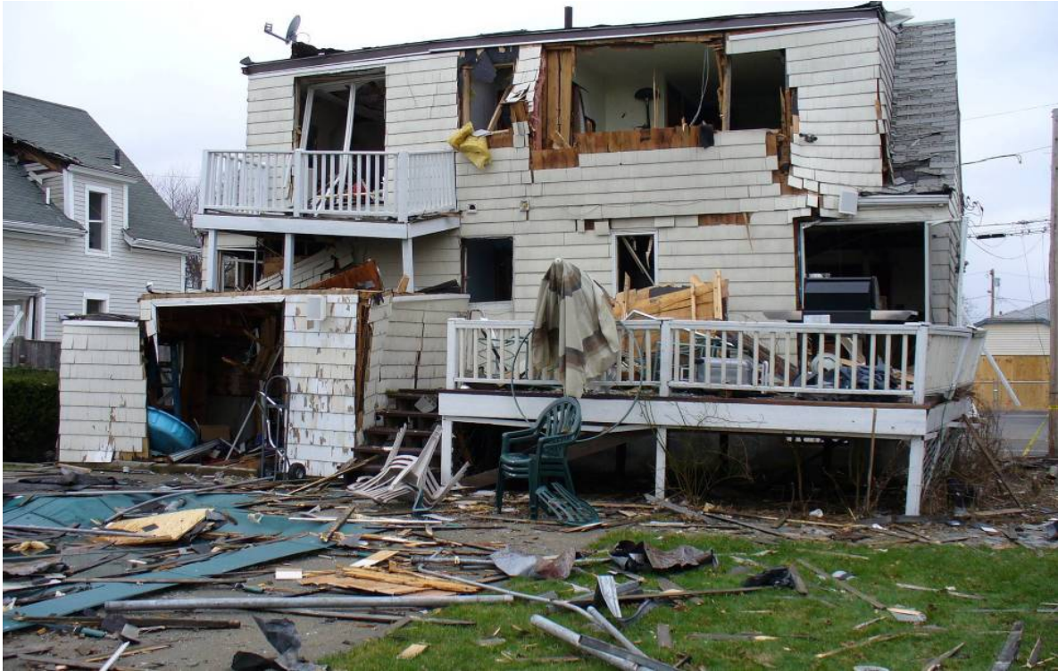
Figure 15. Bates Street home 150 feet north of CAI/Arnel facility destroyed by the explosion.
