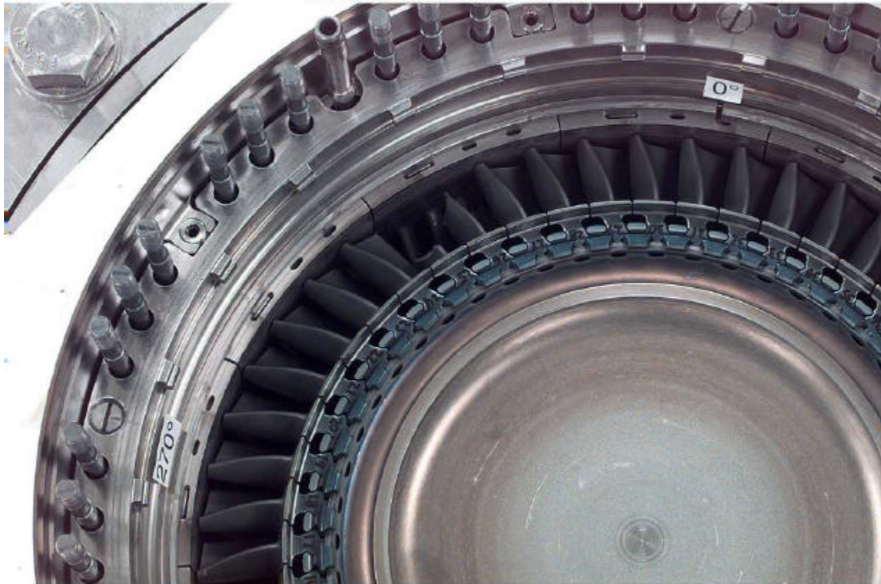
Damaged Turbine Blades (3-4b)
