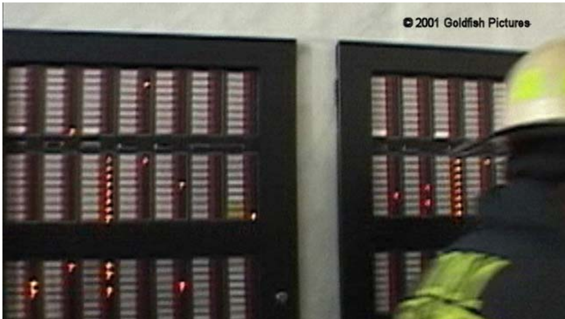
Figure 4–10. Fire alarm system displays at the FCS in WTC 1 showing conditions speaker and telephone circuit faults existing in WTC 2.
