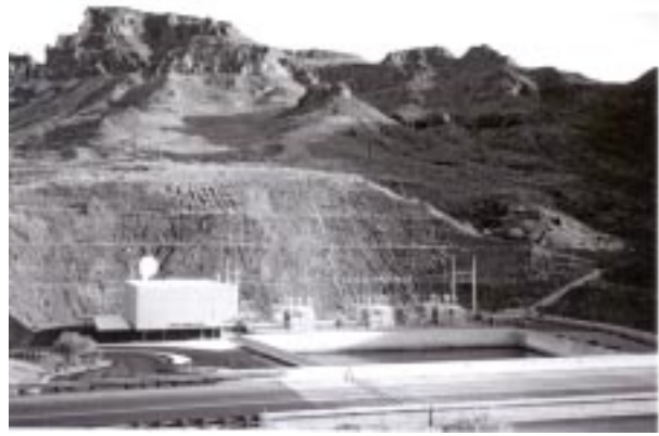
Fig. 38. Colorado River water is lifted nearly 800 feet by the Lake Havasu Pumping Plant located on Lake Havasu near the confluence of the Bill Williams River.
