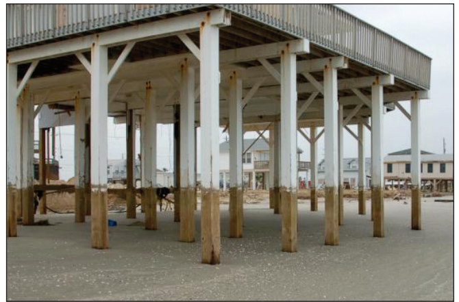
Figure 3. Storm-induced erosion beneath an elevated coastal building (Galveston Island, TX, Hurricane Ike).
