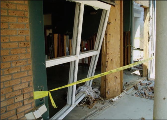
Figure 2. Failure of wood-frame wall, brick veneer, and windows as a result of 4' of stillwater flooding and small waves (Bay St. Louis, MS, Hurricane Katrina).
