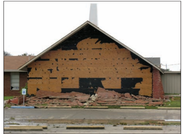
Figure 1. Failed brick veneer over plywood. Many of the ties are still attached to the substrate, but several of the tie fasteners pulled out of the substrate and the ties are embedded in the collapsed veneer. Estimated wind speed: 107 miles per hour (peak gust, Exposure C, at 33 feet).
