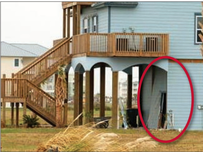
Figure 4. Coastal A-zone flood conditions are sufficient to cause failure of solid breakaway walls and garage doors (west Galveston Island, TX, Hurricane Ike).
