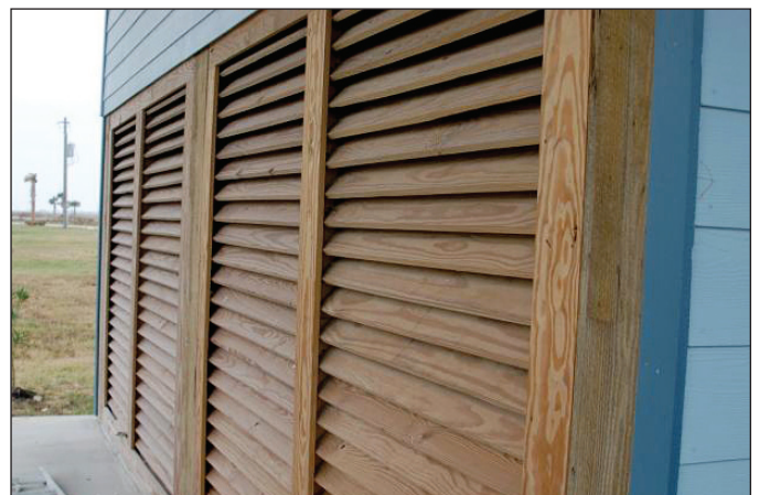
Figure 1. Wood louvers installed beneath an elevated house in a V zone are a good alternative to solid breakaway walls.
