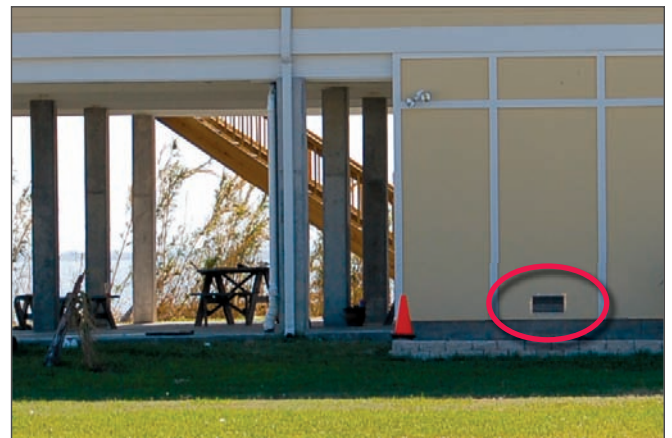
Figure 5. Flood opening in a below-BFE enclosure wall.
