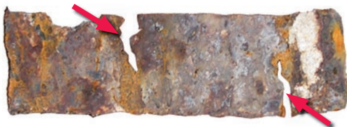
Figure 3. Significant tie corrosion caused the brick at a fire station to fail, even though the building is not near the coast. Note that metal is missing for half of width of the tie at two locations (red arrows). The left end of the tie was still embedded into a concrete masonry unit back-up wall. The right end is where the tie failed in tension, thus leaving a portion of the tie embedded in the collapsed brick.
