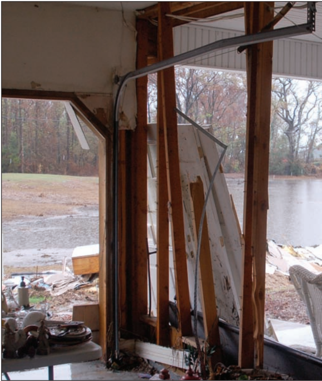
Figure 6. Damage attributed to small waves and approximately 5' of stillwater depth (Bridge City, TX, Hurricane Ike).
