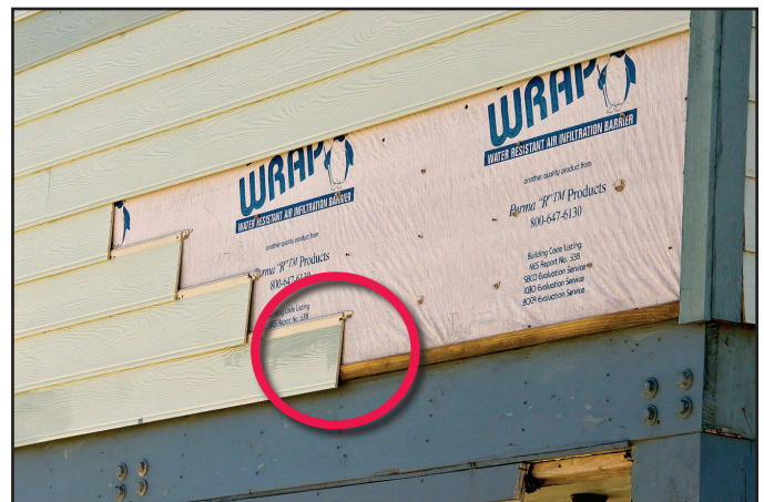
Figure 12. Blind nailed siding installed with exposed gap at bottom (red circle) is vulnerable to failure.
