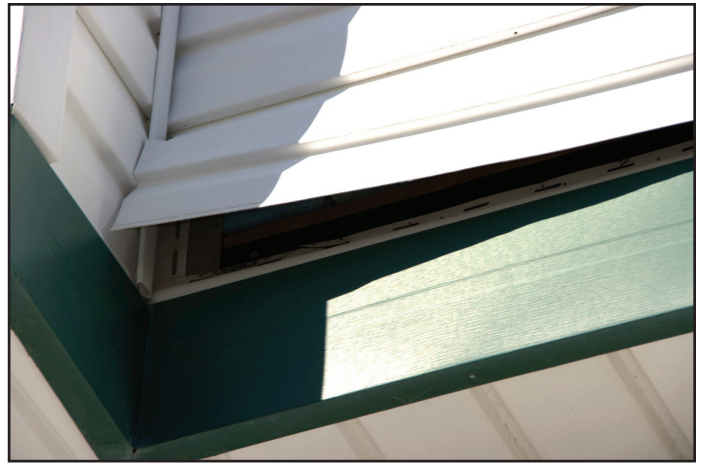
Figure 4. Utility trim was substituted for the starter strip and the bottom lock was cut off the siding. Siding was able to pull loose under wind pressure.
