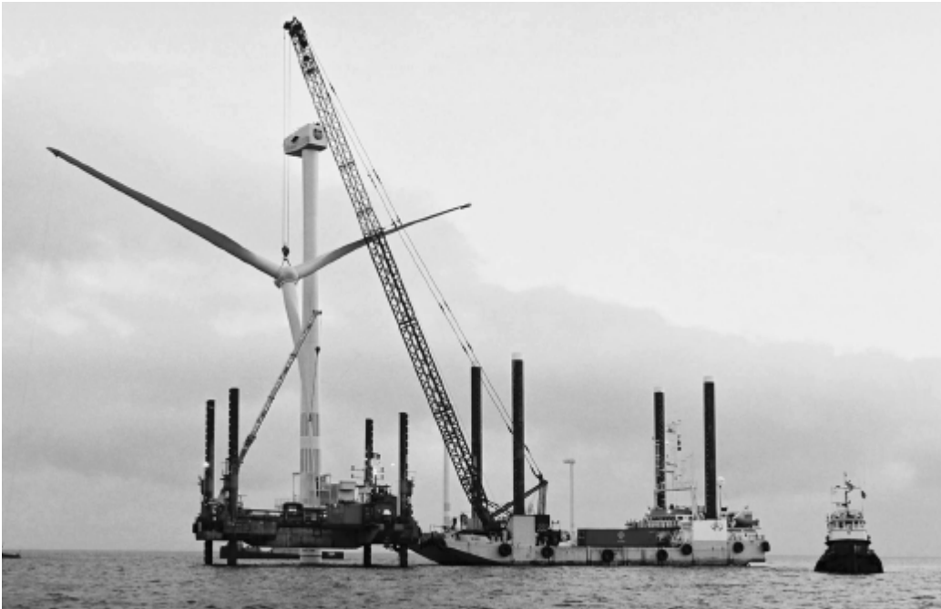
Figure 21.6 Utgrunden Offshore 10-MW wind farm
