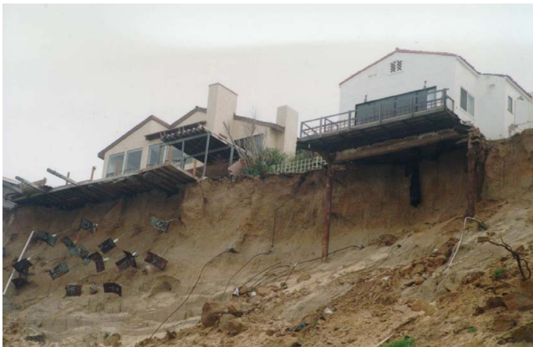
Figure D.4.6-29. Bluff Failure and Retreat, Encinitas, California (Photo by Noble Consultants, Inc.)
