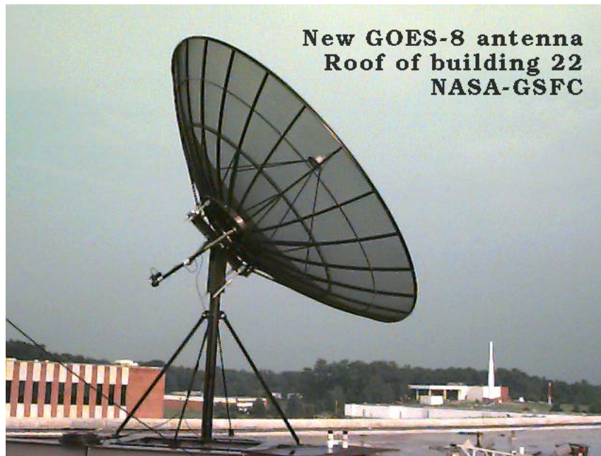
Figure 2: GOES steerable 5-meter S-band antenna on rooftop at NASA-GSFC.
