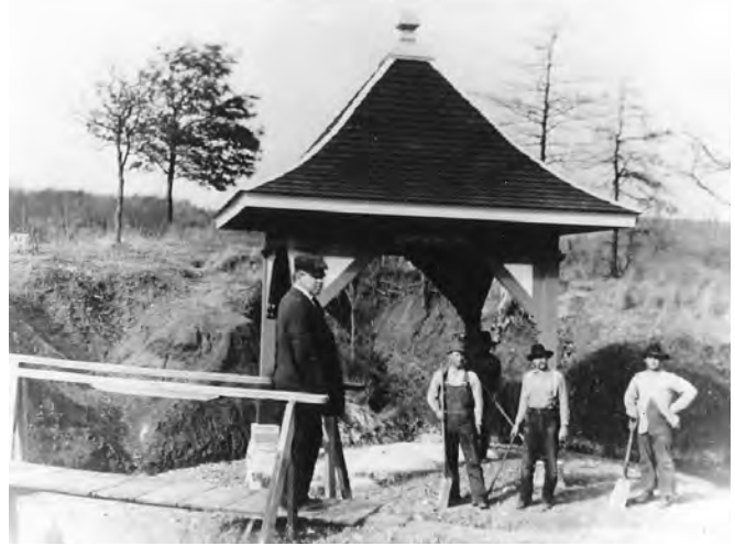
Figure 3-55. Construction of an early pavilion at Black Sulphur Springs in the southern part of the Platt National Park, circa 1915. Note the open prairie landscape behind the workers and the pavilion.
