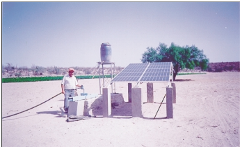
Figure 1: Photovoltaic water pumping system at Rancho Agua Blanca, Baja California Sur, Mexico.
