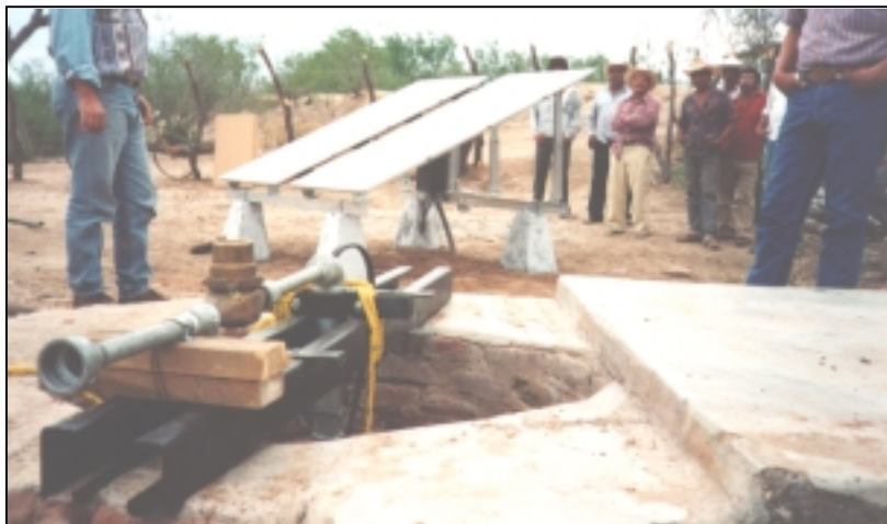
Figure 2: This PV water pumping system was installed in 1994 in the rural community of Sirebampo, Sonora. It produces 5,000 liters of water per day from a hand dug well equipped with a submersible centrifugal pump powered by 8 PV modules (424 Watts).
