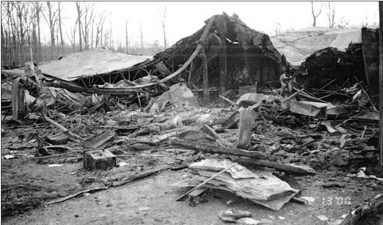
Figure 10. View of collapsed truss and accordioned support column (left side of picture).
