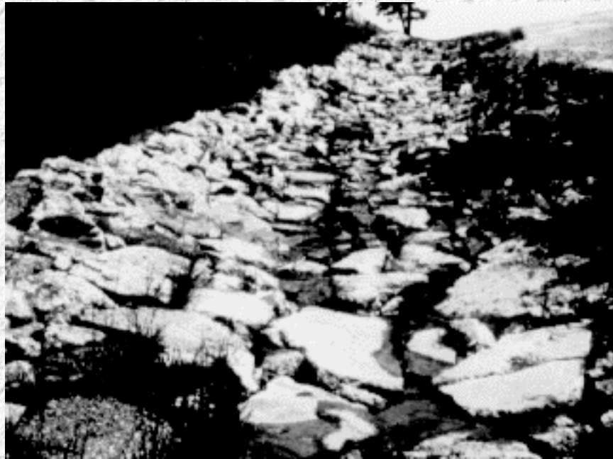
Figure 8. Broken Concrete Riprap
