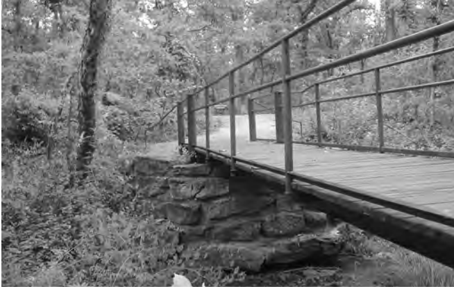
Figure 6-77. Wood plank and pipe railing bridge situated on revised historic abutments, where steps and stepping stones once existed, 2001.
