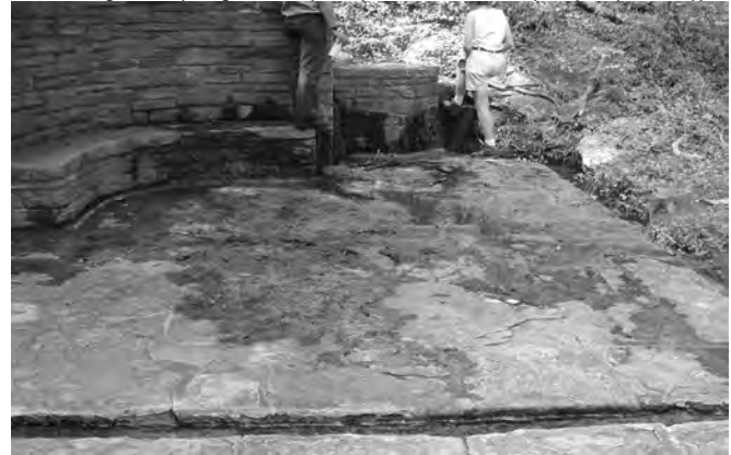
Figure 6-53. Runnel and seepage at Hillside Springs terrace, 2002.
