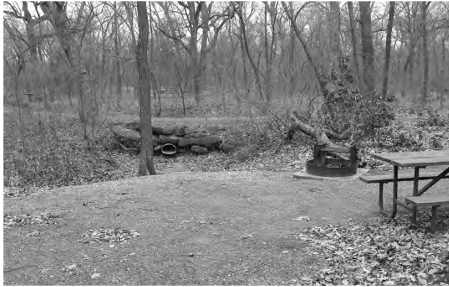
Figure 6-86. Culvert headwall just north of Chigger Hill area of Rock Creek Campground, 2004.
