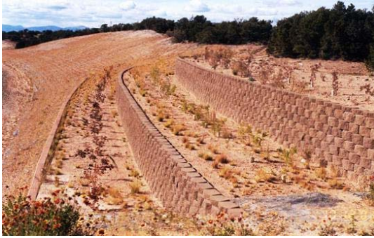
Figure 12: Northwest quadrant near the conclusion of the first growing season on New Mexico Highway 599 at the Ridgecrest Road Interchange (November 2001)
