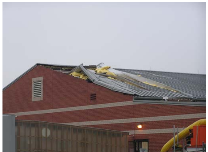
Ashland County Tornado Damage August 9th, 2007 NWS photo
