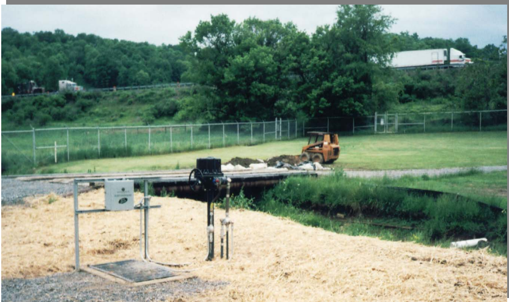
Autonomous Spill Detection Sensor Over Grated Sump Remote Gas Compressor Station, West Virginia
