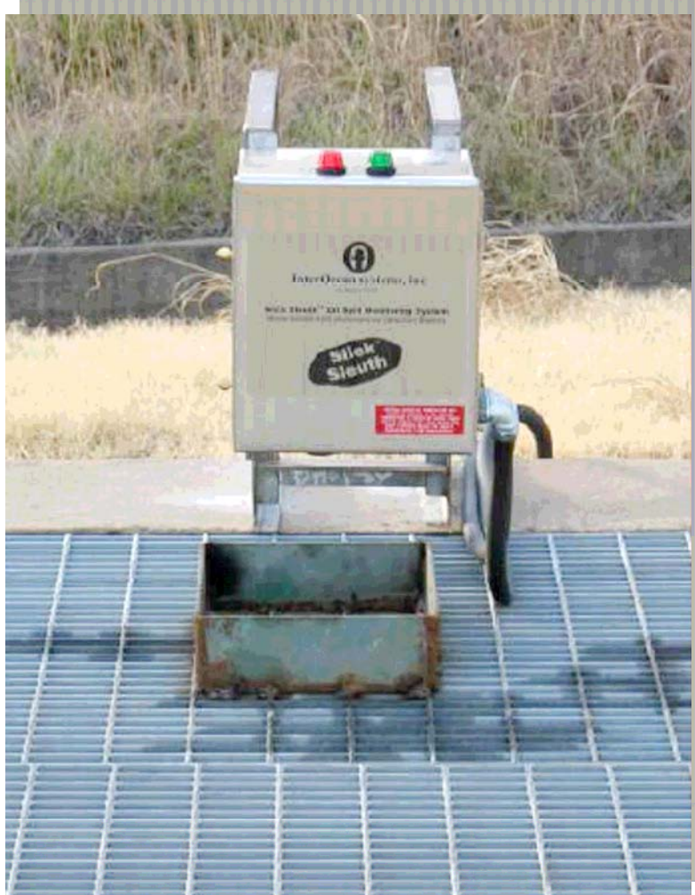
Autonomous Spill Detection Sensor 'Peering' Down Into Deep Pit Sump at GenCo (photo courtesy of Entergy, Arkansas)
