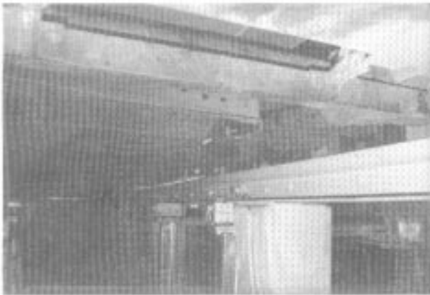
Figure 71. Munich maintenance shop (photo—showing traction motor and shop pit with sliding rail for traction motor drop).
