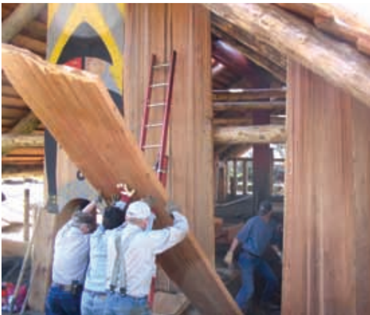
A crew of three volunteers positions a cedar plank for the Cathlapotle Plankhouse at Ridgefield NWR (Washington). (Photo U.S. Fish & Wildlife Service)
