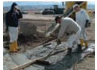
Volunteers pour and finish a cement walkway at Lee Metcalf NWR (Montana). (Photo U.S. Fish & Wildlife Service)
