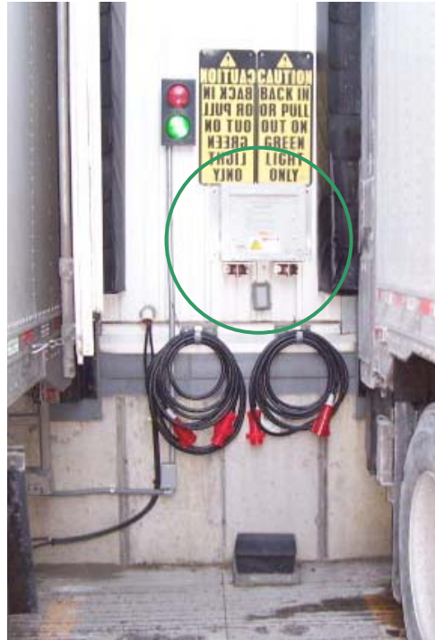
Figure 3-7: Warehouse-Mounted Electrical Power Module
