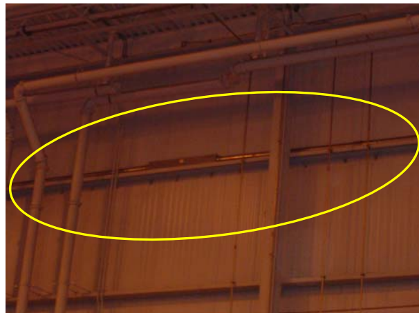
Figure 3-2: Warehouse Installation of Conduit Containing 300 Amp 3 Phase 480 VAC Power (2 of 2)
