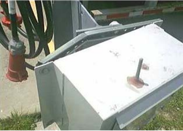
Figure 5-8. Top View of Pedestal 2 after Collision with Trailer
