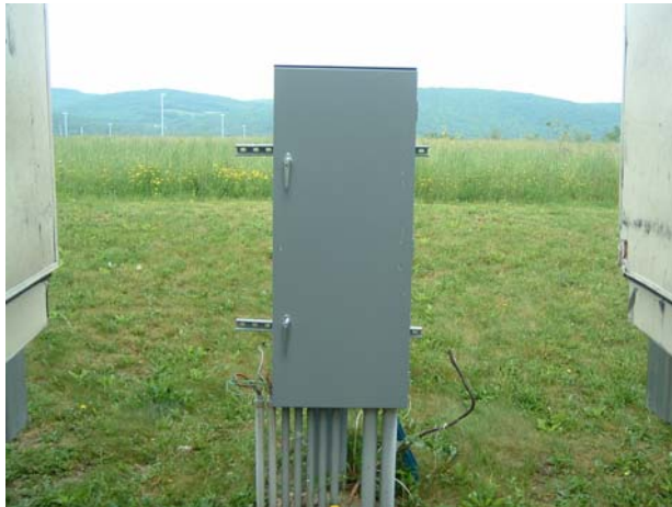
Figure 3-5: Electrical Facility Installation – 300 Amp 480 VAC 3 Phase Breaker Panel
