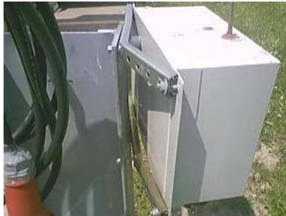
Figure 5-9. Side View of Pedestal 2 after Collision with Trailer
