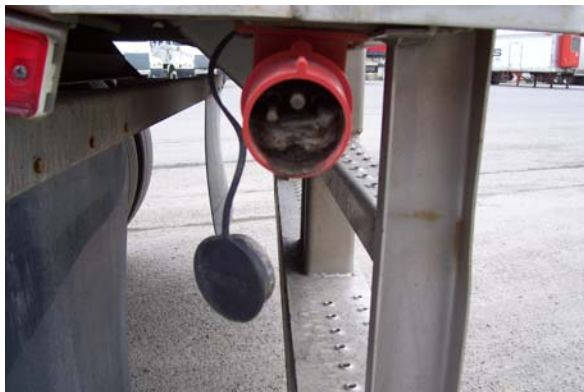
Figure 5-4: Front View of Original Plug Mounted on TR350
