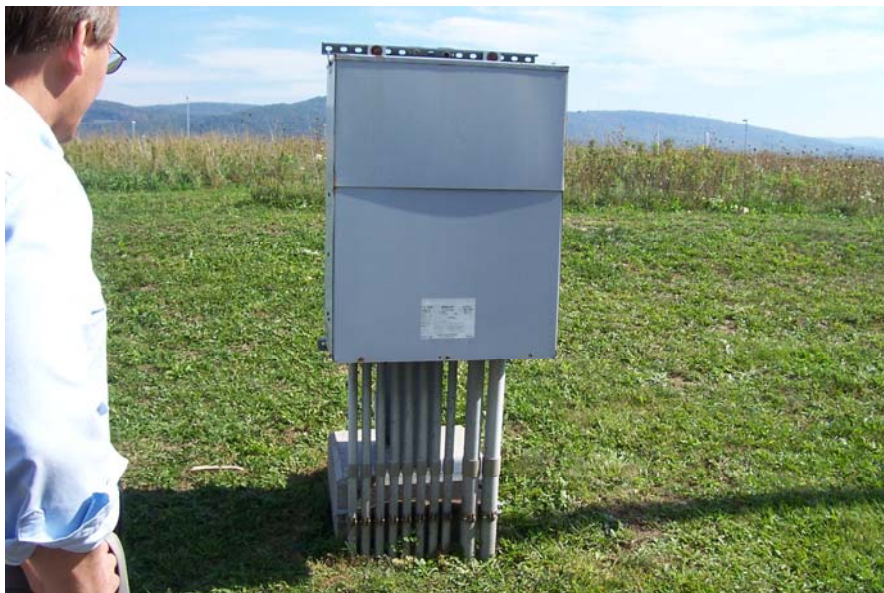
Figure 2-3: Existing Electrical Distribution Panel in Trailer Parking Lot
