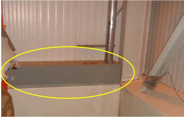
Figure 3-3: Warehouse Installation of Conduit Containing 300 Amp 3 Phase 480 VAC Power – Junction Box to 2 Inch Conduit
