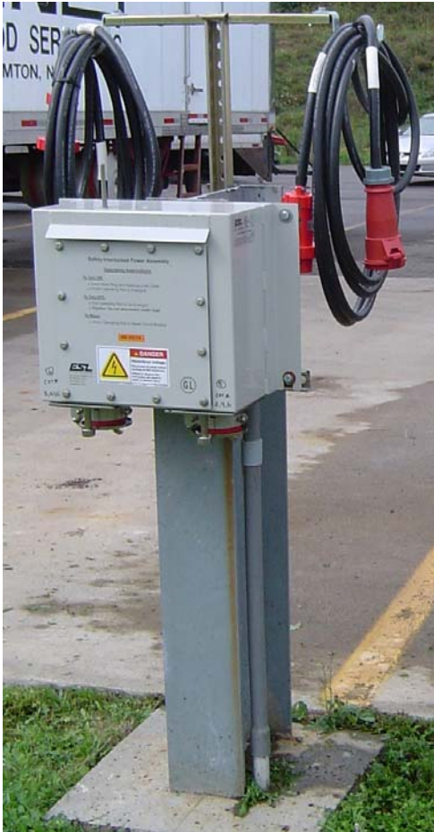
Figure 3-6: I-Beam-Mounted Electrical Power Module
