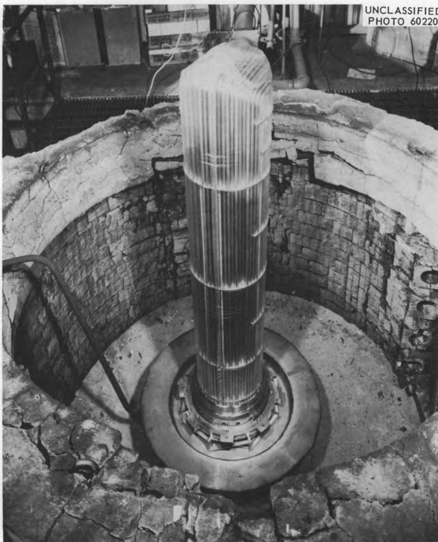
Fig. 13. Tube Bundle Positioned in Furnace Pit on Retort Base with Protective Bag Still in Place.
