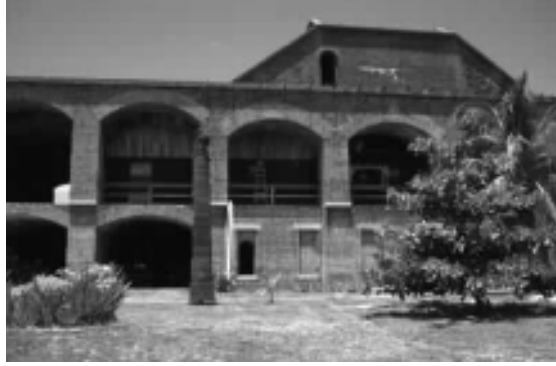
A prototype housing unit was completed. Its roof and wall systems are independent of the surrounding casemates of Fort Jefferson.
