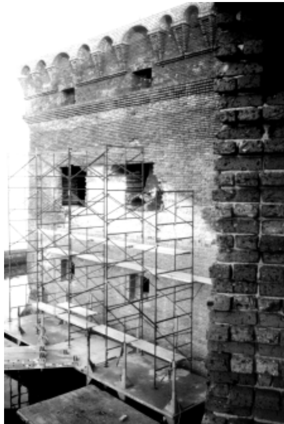
Stabilization work on the fort's southwest bastion is part of ongoing efforts to preserve the structure and prevent further deterioration.
