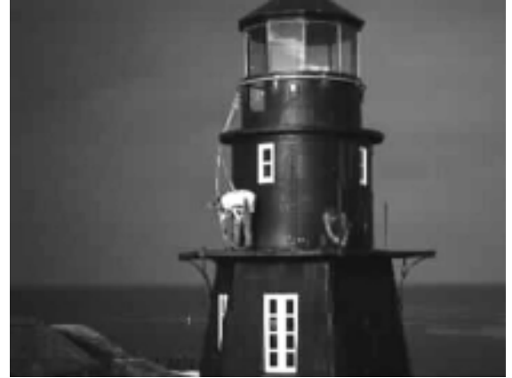
Extensive repairs and preservation work on the Garden Key harbor light raised the structure's condition to "good".
