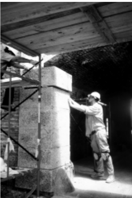
Masons disassemble granite sally port arch to remove iron hinges at base.
