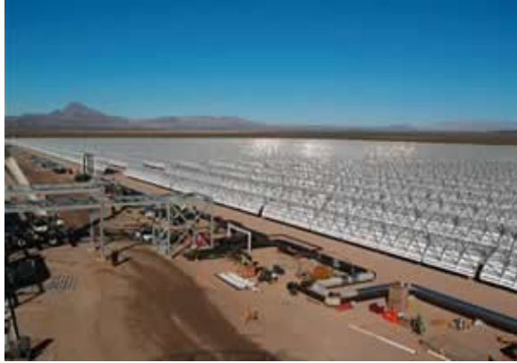
Figure 2.2 Nevada Solar One Solar Thermal Plant Courtesy of Solargenix Energy
