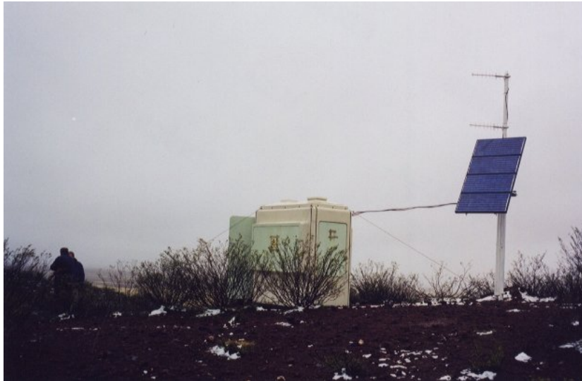
Figure 3.4.5 : Los Leones base-station controller shelter (Dec 1999 - May 2001)
