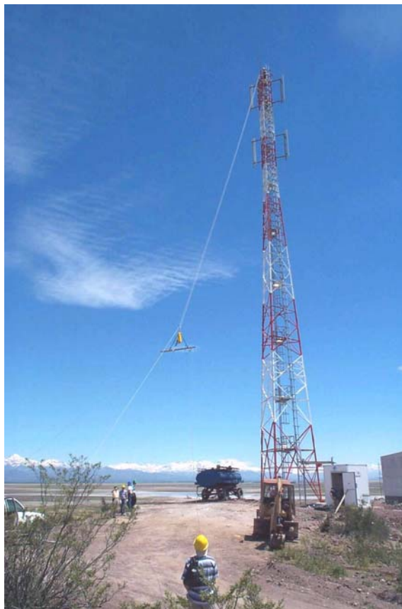
Figure 3.1.6: Installation of WLAN panel antennas on the 41 metre tower at Los Leones
