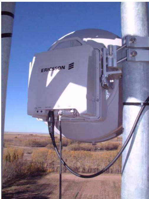
Figure 3.3.1 : Dish-mounted microwave radio on the campus tower
