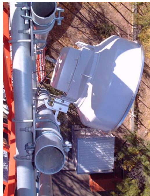
Figure 3.3.2 : Top view of 0.6m diameter microwave dish and radio unit
