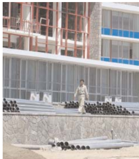
Workman finishing up the large new dormitory for women at Kabul University built by USAID. The univer-
