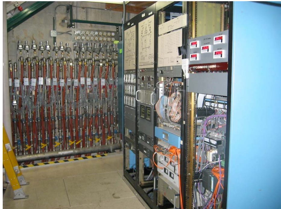
The 210 neutral beamline water manifold and local control station
