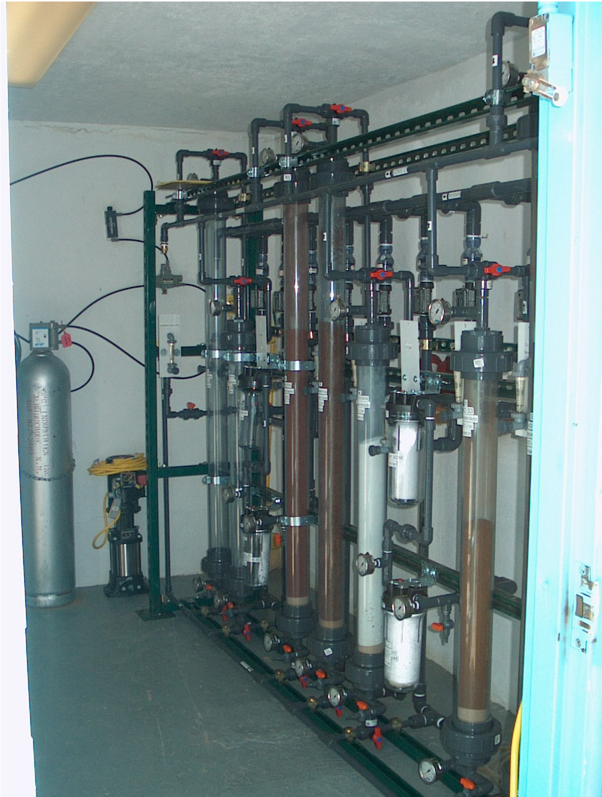
Figure 3-1. Socorro Springs Pilot Skid Unit.
