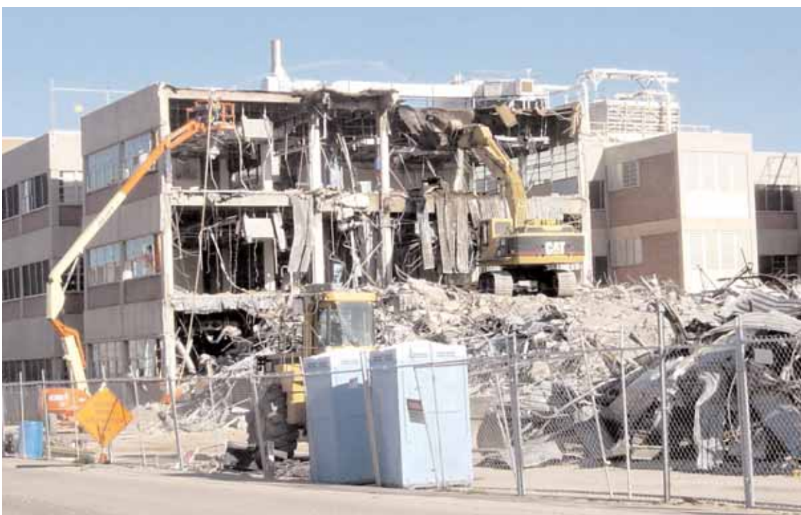
DOWN IT COMES — Building 805, which combined office and laboratory space and was home to many Sandians for many years, comes down under the experienced hand of Coronado Wrecking.
