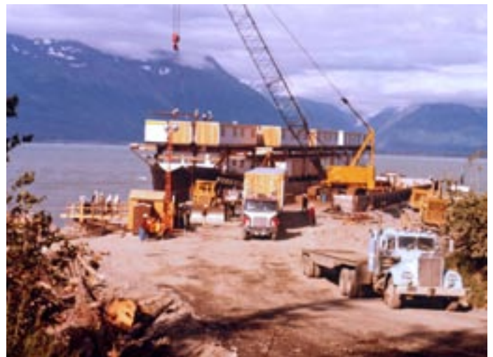
(center) Pipe came by the truckload in 40 foot and 60 foot lengths and weighed 235-285 pounds per foot.
