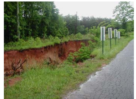
Ridge Road before treatment.
