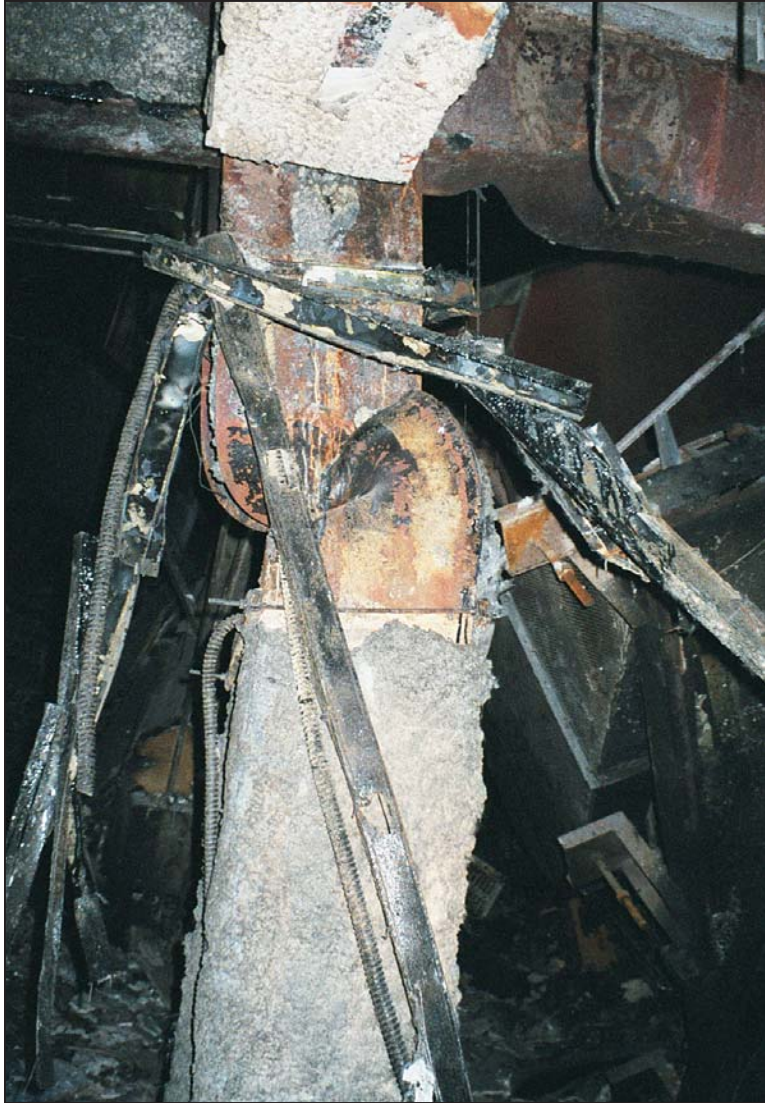
Figure 4-17 Buckled beam flange and column on the 8th floor of WTC 5 that was weakened by fire.
