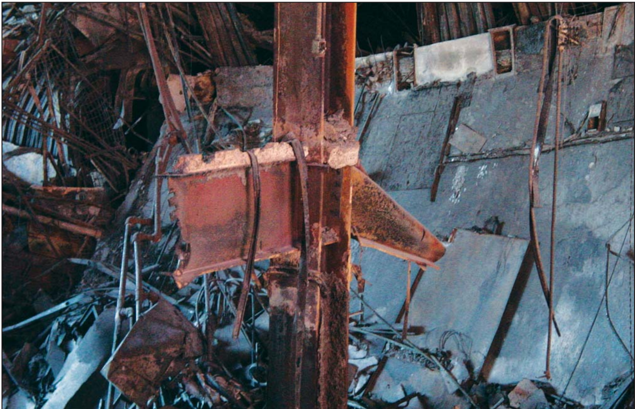
Figure 4-21 Internal collapsed area in WTC 5 with closeup of connection failure at column tree.
