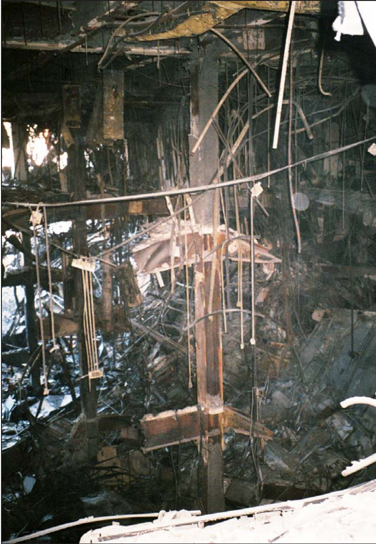
Figure 4-19 Internal collapsed area in WTC 5.
