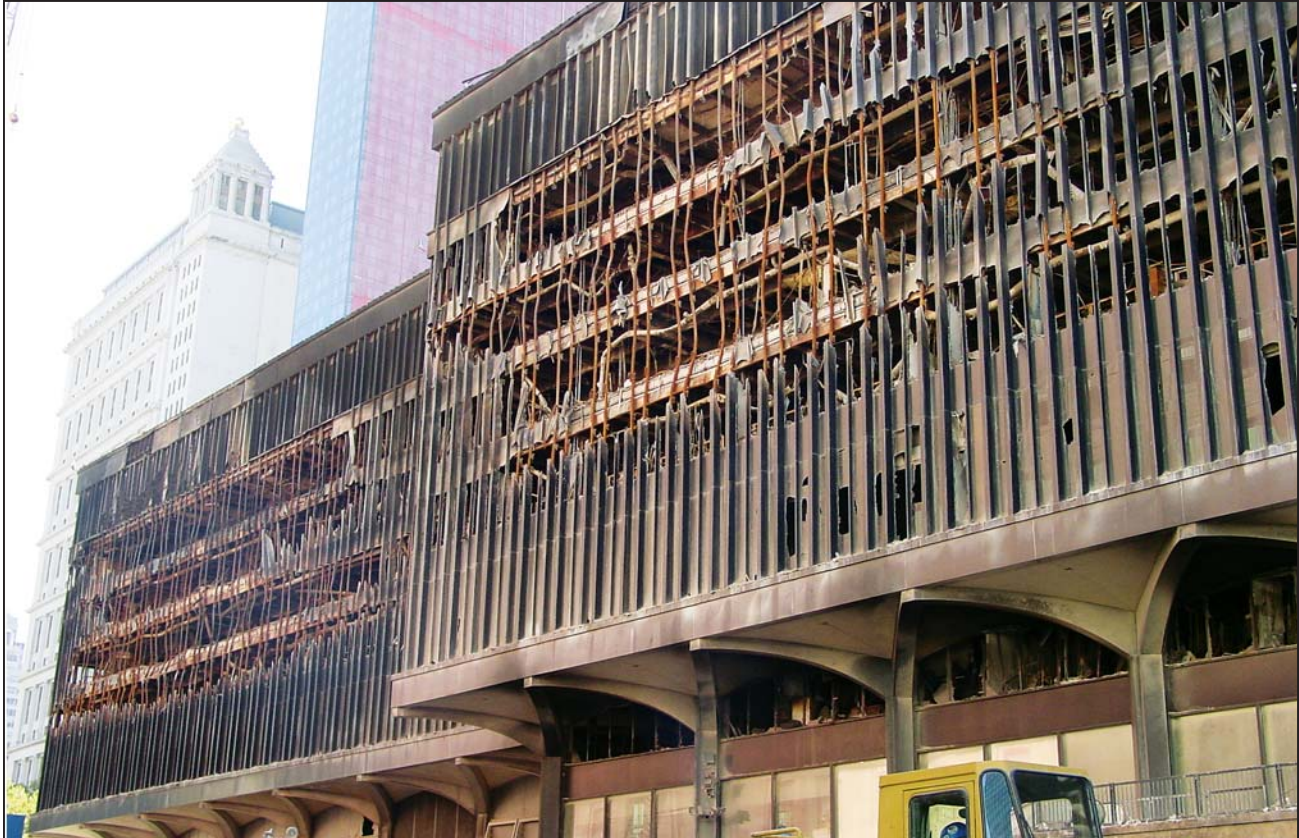
Figure 4-11 WTC 5 façade damage.
