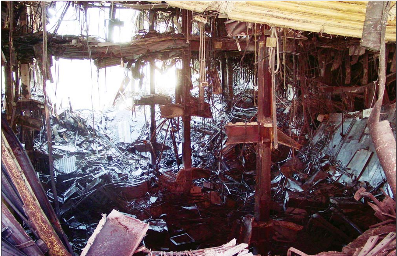
Figure 4-20 Internal collapsed area in WTC 5.
