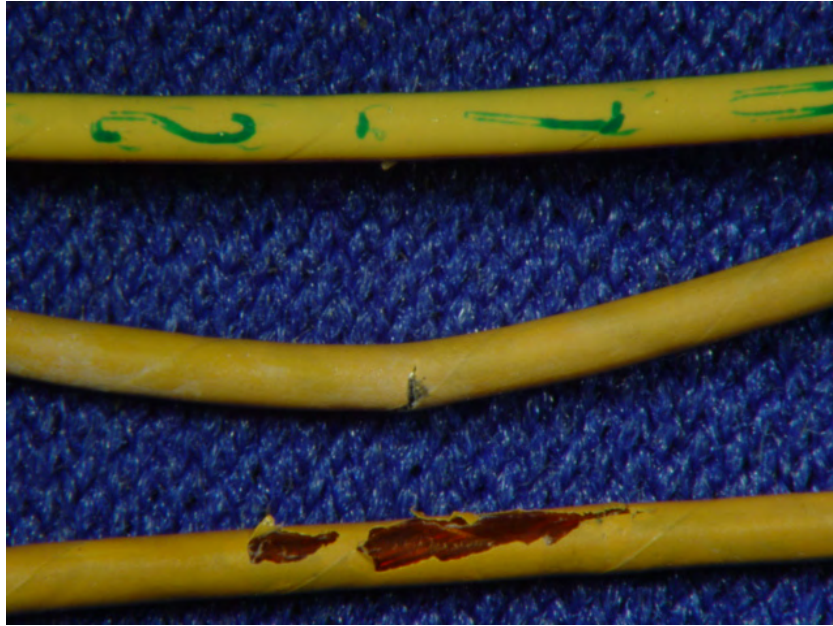
Figure 14. Progression of Insulation Damage, Aged at 250°C
