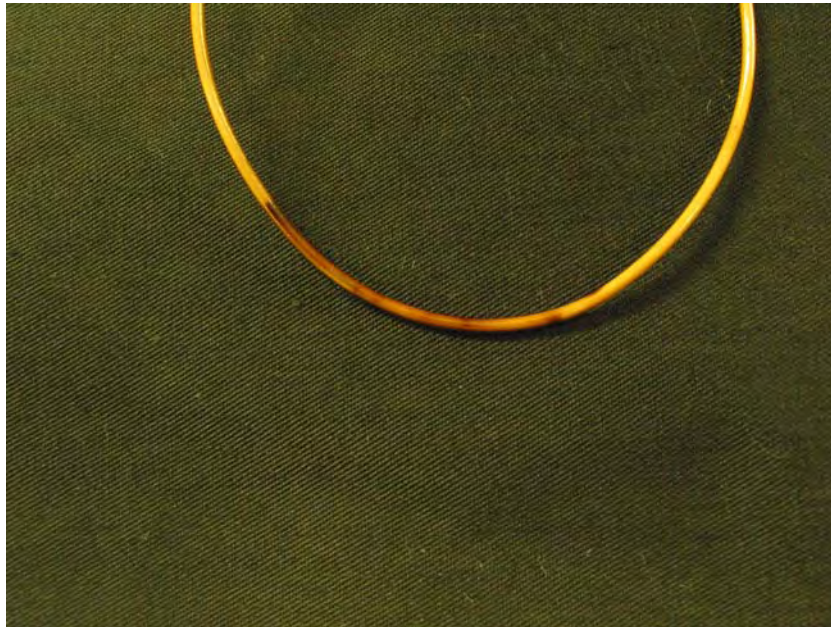
Figure B-1. Localized Discoloration on PV Wire
