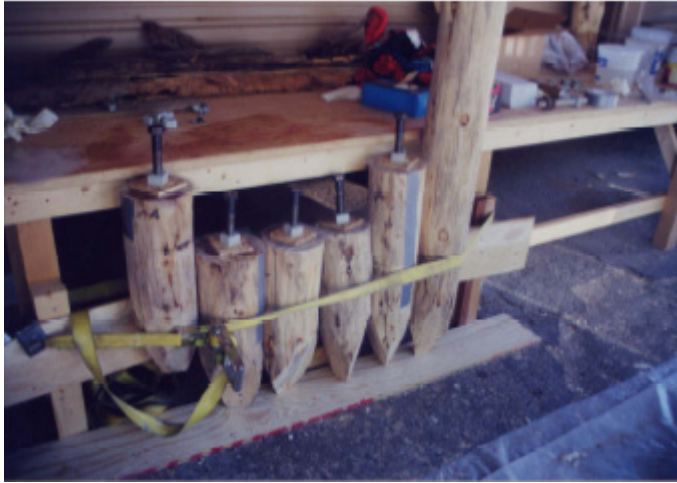
New viga ends after temporary insertion of threaded rods to create threaded mold.
