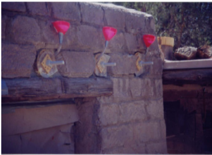
Existing viga ends with temporary epoxy filler tubes and permanent threaded rods installed.
