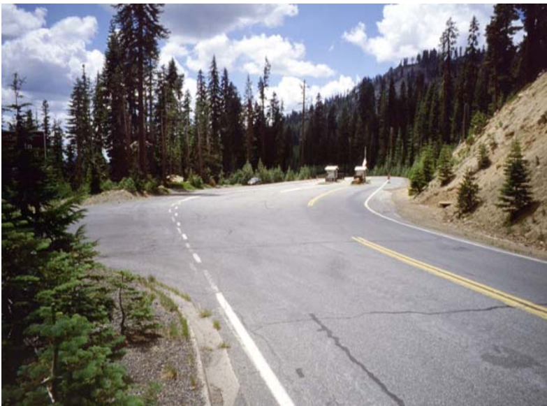
DETERIORATED CURBING, ASPHALT AND POOR DRAINAGE
