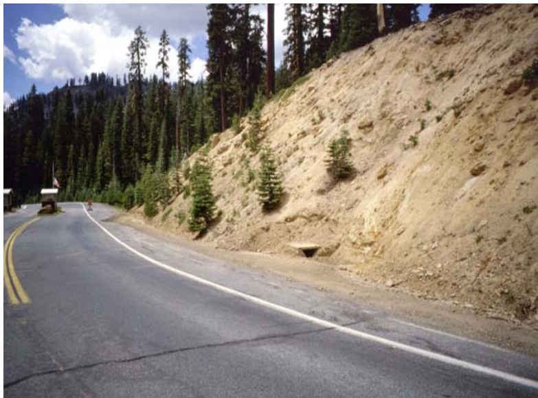
POOR DRAINAGE, SLOPE EROSION ONTO ROAD AND DETERIORATED ASPHALT
