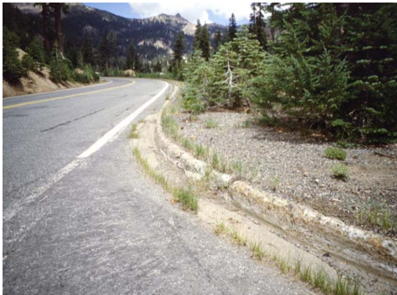
DETERIORATED CURB AND ASPHALT
