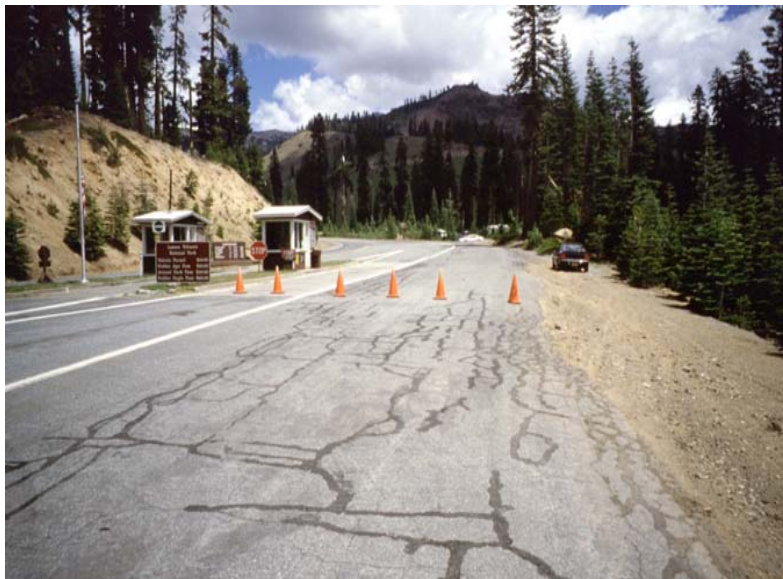
CRACKED AND DETERIORATED ASPHALT
