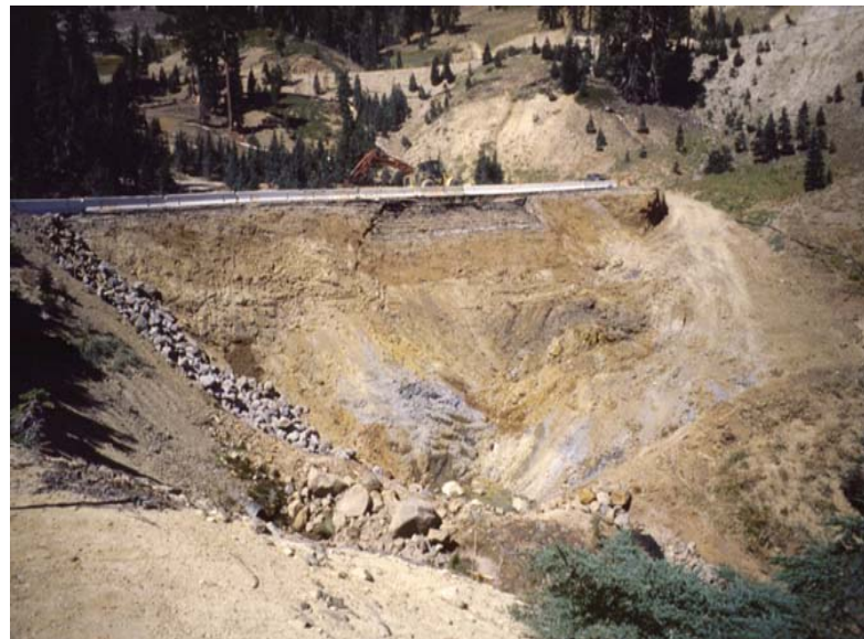
SLIPOUT DURING EXCAVATION
