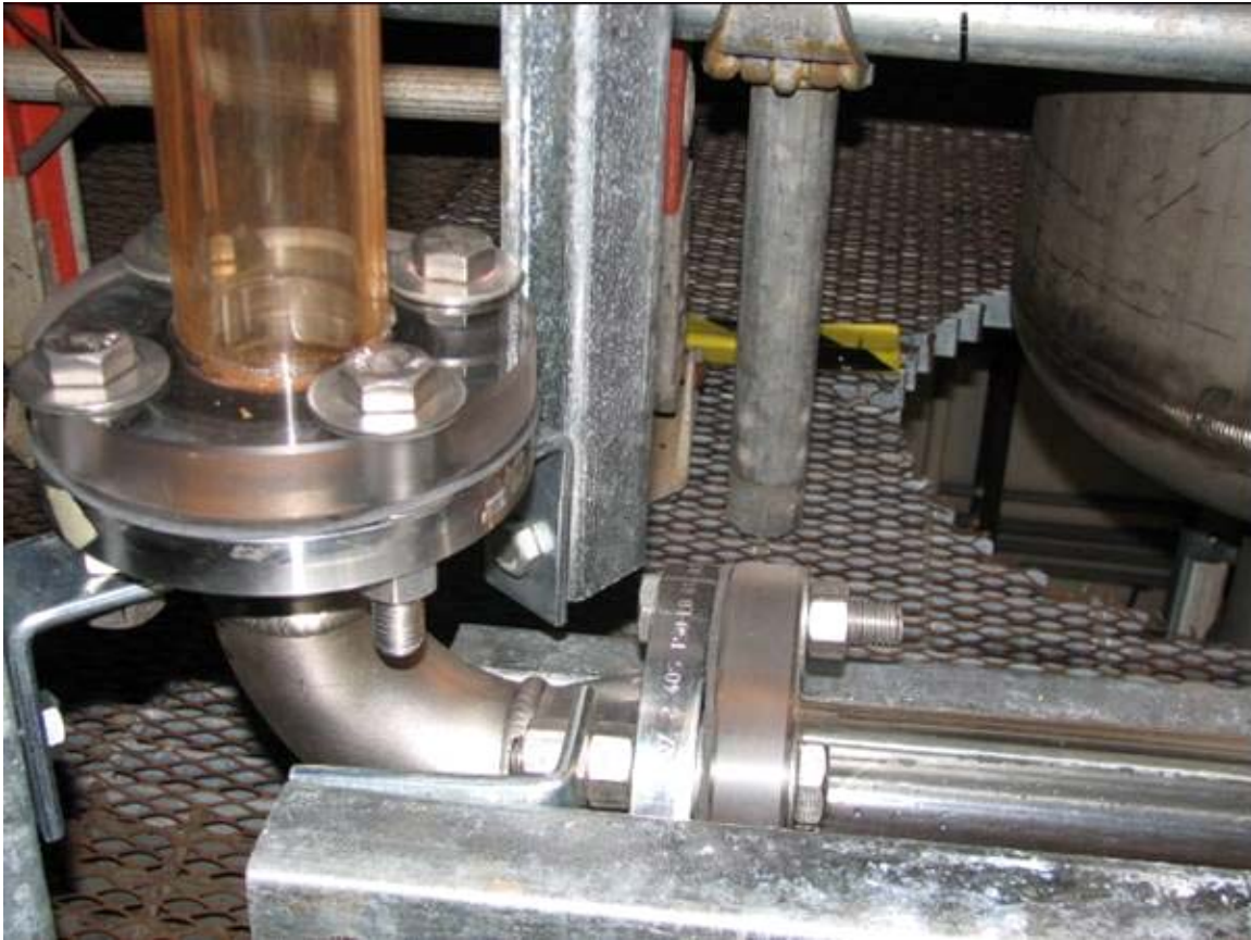
Figure 21. Third Clear Section After 400 Cycles of AZ-101, Test 15
