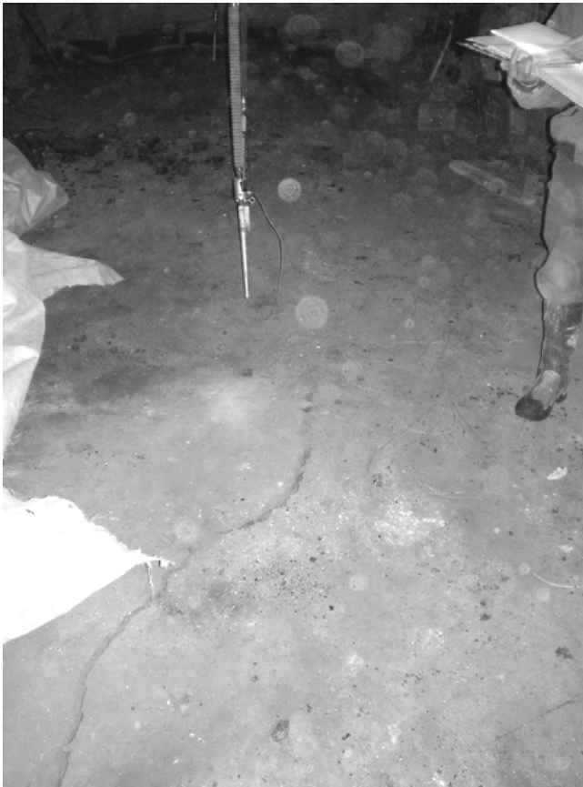
Figure 9. Floor heave located approximately in the middle of recovery chute C.
