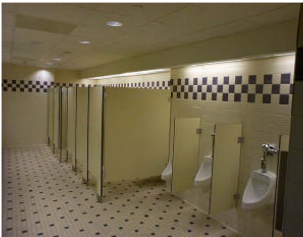
New low-flow plumbing fixtures and efficient lighting in the Pentagon bathrooms.
