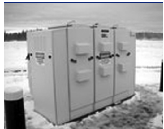
Figure 1. Fuel cell model installed.*
