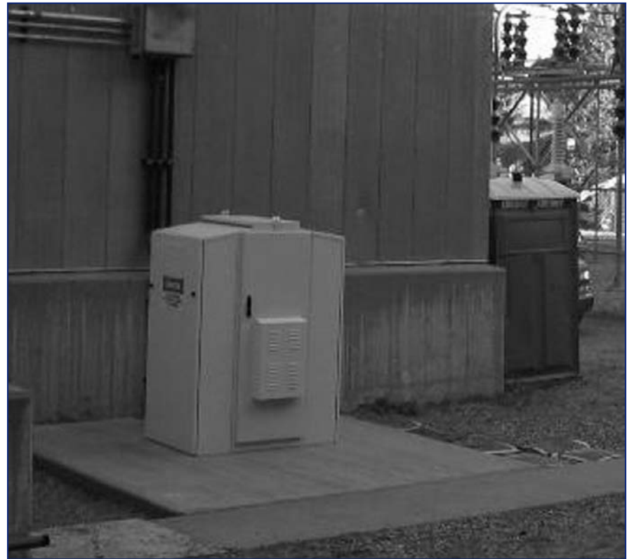
Figure 4. BOR fuel cell model installed.
