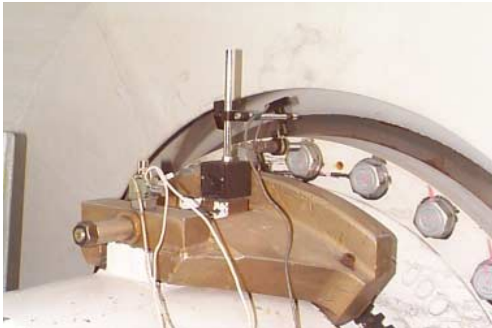
Figure 8. Triaxial accelerometer sensor on low-speed shaft bearing
