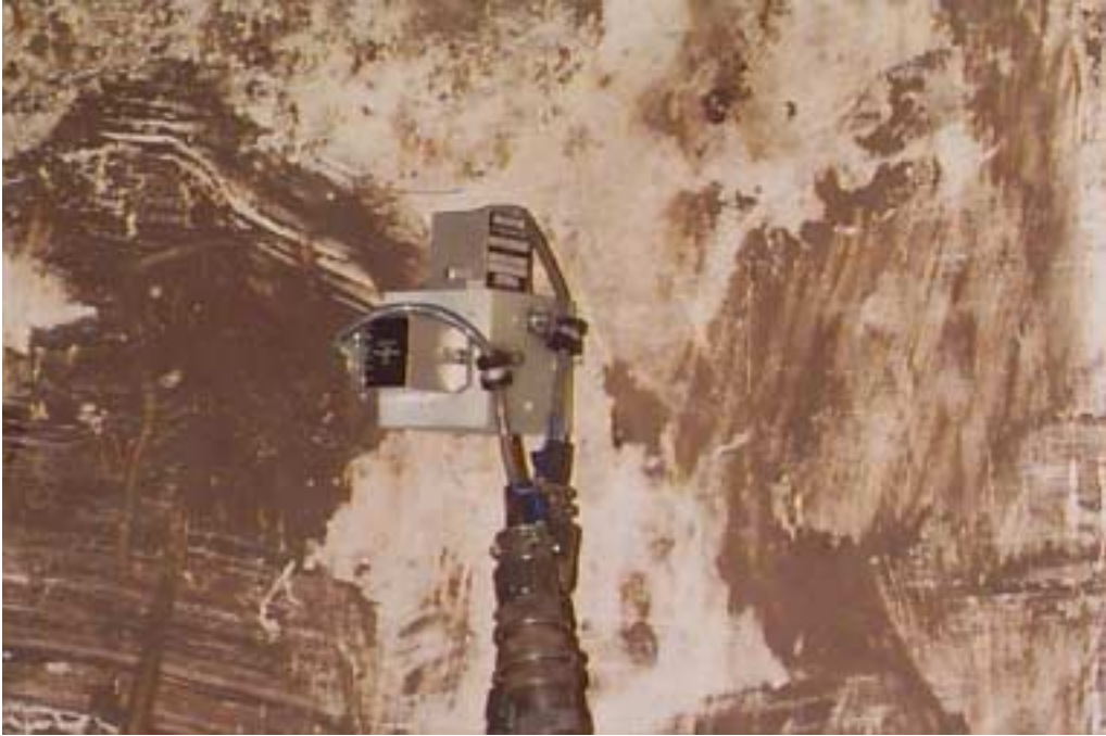
Figure 9. Biaxial accelerometer mounted inside tower below yaw bearing
