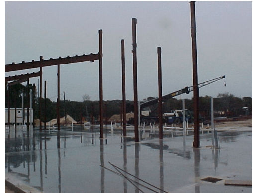
Girders rise from the floor of the Environmental Education Center in the GTM NERR
